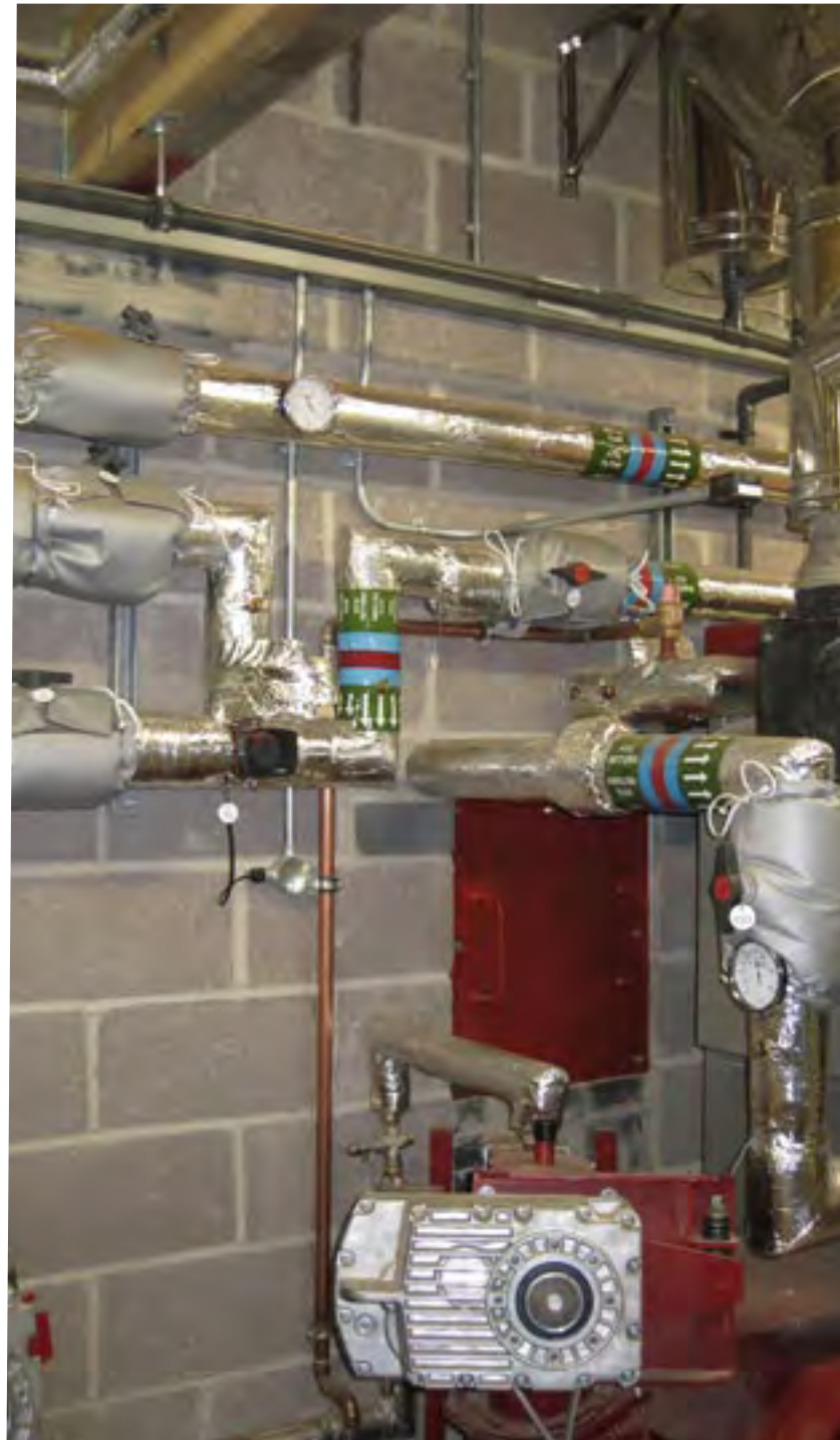
Biomass boiler | Uppark House and Garden
