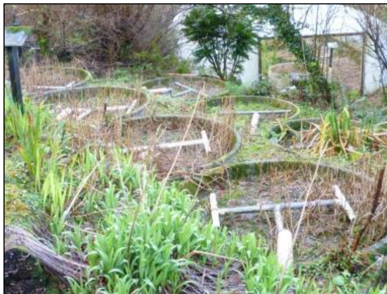
Second stage of the reed bed system for the eco cabins
